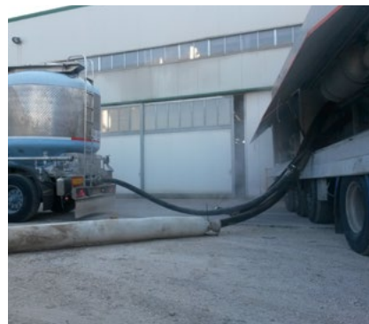
Pneumatic refilling system for cement compartment
