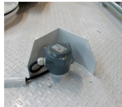
Level sensor on the cement compartment
