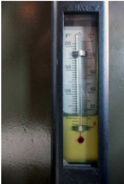
Fig. 6.4-1 - Hydraulic oil tank level visual indicator
